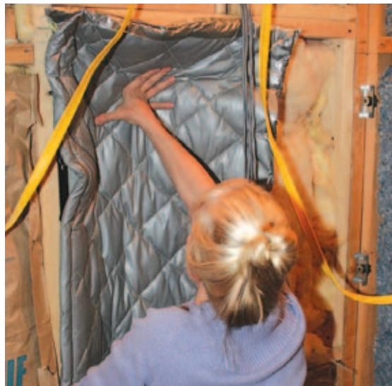
Figure 8. Most dedicated home theaters have built-in speakers. To contain noise and low-frequency vibrations, the author often lines the cavity behind the speakers with a special quilted fiberglass insulation that contains a high-density loaded-vinyl barrier.
