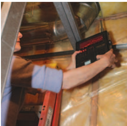
Figure 11. Acoustic treatments should always be tested before drywall is installed. The author uses a tone generator and graphic sound analyzer to measure the decibel level at specific frequencies. If the required STC is not met, she takes additional measures.
